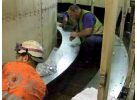
Installation of a guide trough in a circular path for an indoor / outdoor loop
