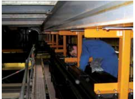
Mounting in an electroplating plant in cramped conditions
