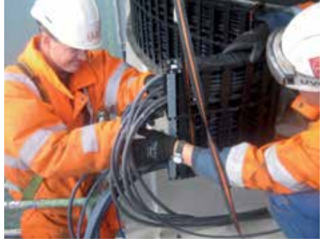
Equipping a crane's swivel beam with an e-chain® for rotating motion
