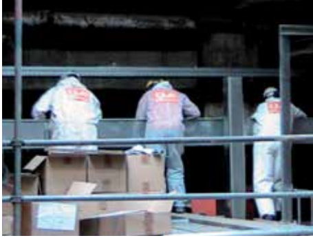
Updating a trailing cable system for Rol E-Chain® in a waste bunker crane
