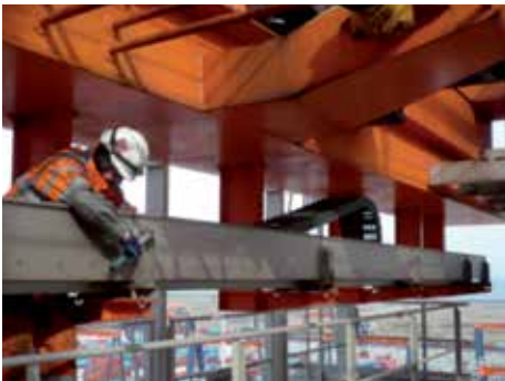
Installation of an e-chain system® and guide trough on a ship-to-shore crane
