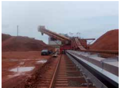
Replacing the chain's covered trough, which protects the system from the weather
